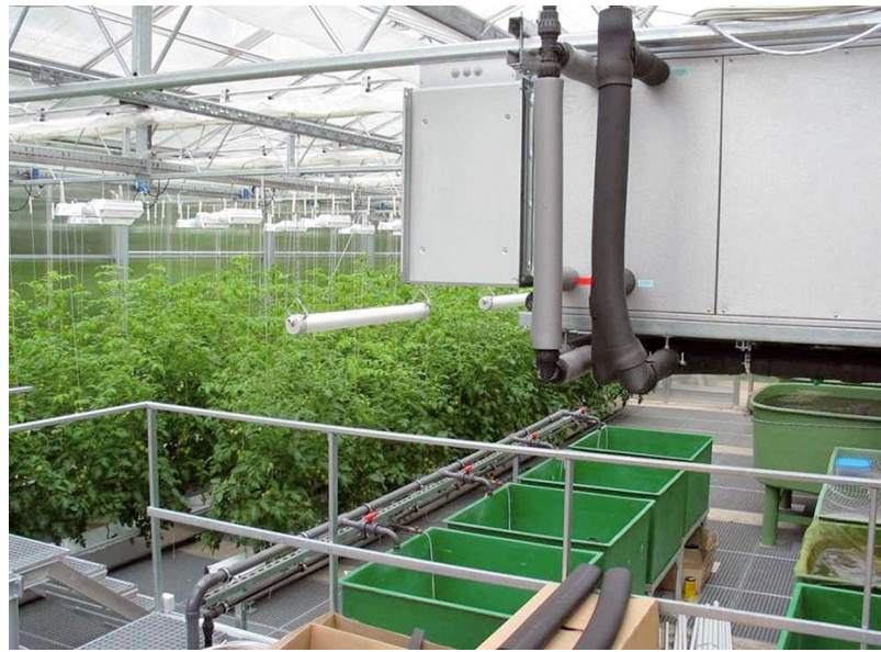
Fig. 2. ASTAF-PRO prototype during the test period in early April 2009, showing aquaculture fish tanks (green boxes) containing tilapia ( Oreochromis niloticus ) and hydroponic troughs with tomato plants Solanum lycopersicum and the air-conditioning system
